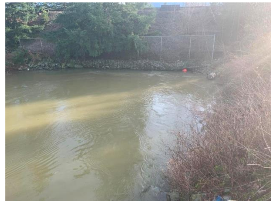
Culverts nearly plugged
